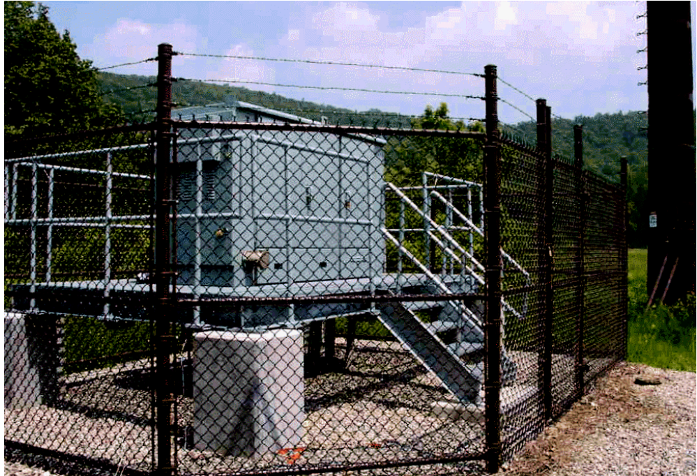
FIGURE 3-4 TYPICAL OUTDOOR ENCLOSURE CABINET ON RAISED PLATFORM
